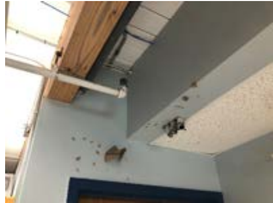
Upright Sprinkler – Soffit Obstruction
