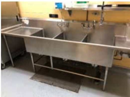
Scullery Sink w/Recessed Grease Interceptor
