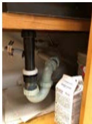
Lab Waste Piping
