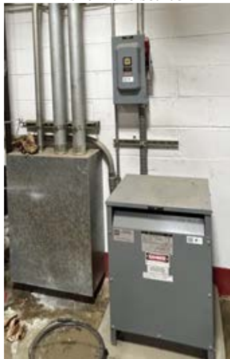
Dry Type Transformer
