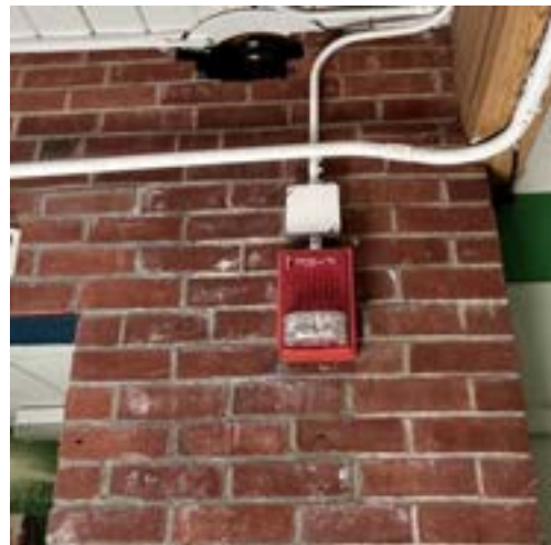
Fire Alarm Annunciator and Device
