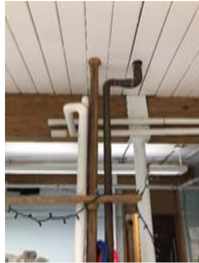
Copper Vent Pipe
