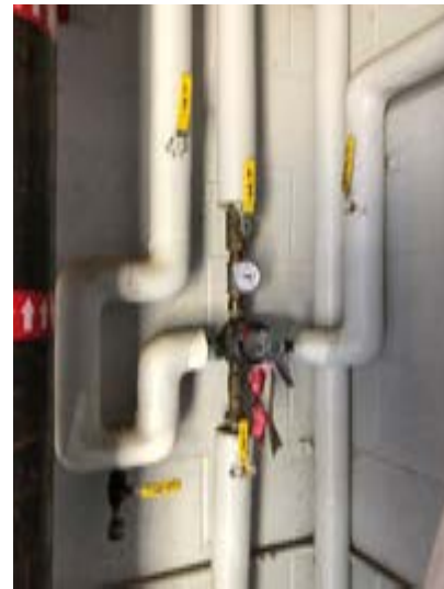
Exterior Mech Room Mixing Valve
