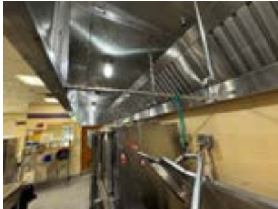
Main Kitchen Type I Exhaust Hood
