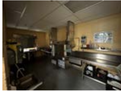
Main Kitchen Type II Exhaust Hood
