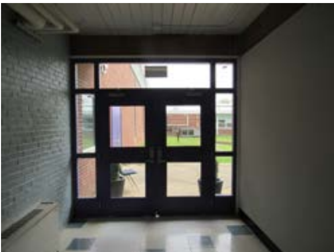
NO PERIMETER DOOR MONITORING.
