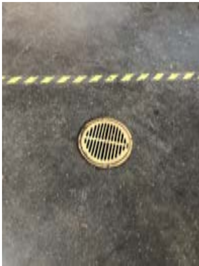
Auto Shop Area Drain
