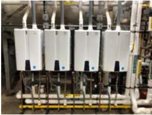
Gas-Fired Water Heaters
