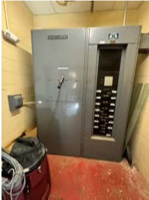
Switchboard #2 (208Y/120V, 1200A)
