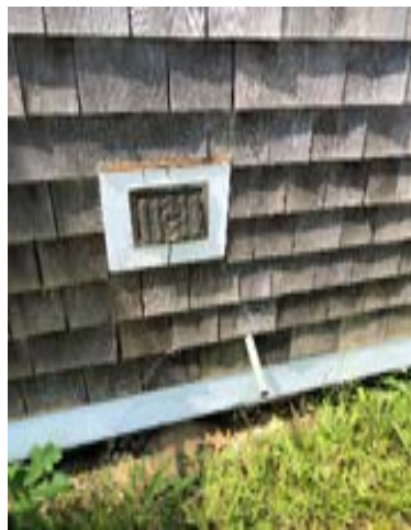
Exterior Wall Hydrant
