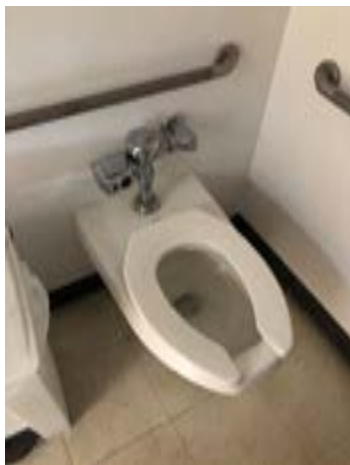
Wall Hung Flush Valve Toilet
