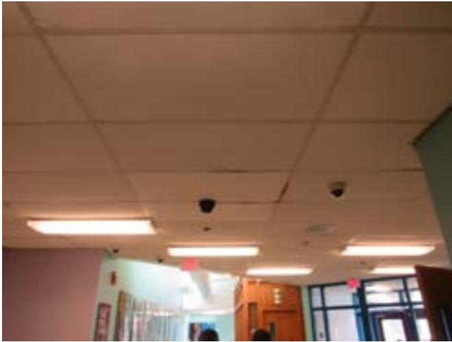
POOR CONDITION OF DROP CEILING AND MULTIPLE CAMERAS AT APEX.
