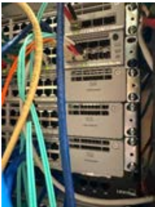
MDF Network Switch Electronics
