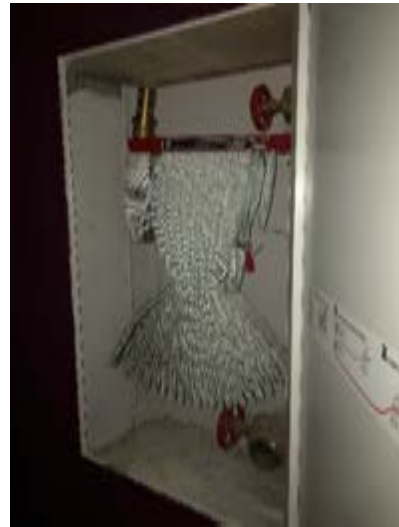
Hose Station at Stage
