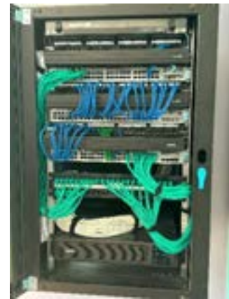
IDF Patch Panels and Electronics
