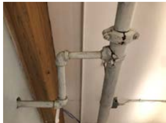
Evidence of Leaks at Grooved Fittings
