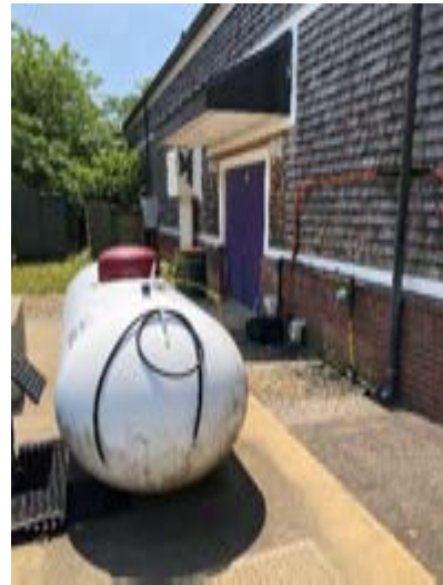
LP Tank and Piping
