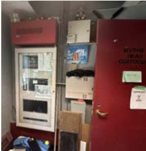
Fire Alarm Control Panel
