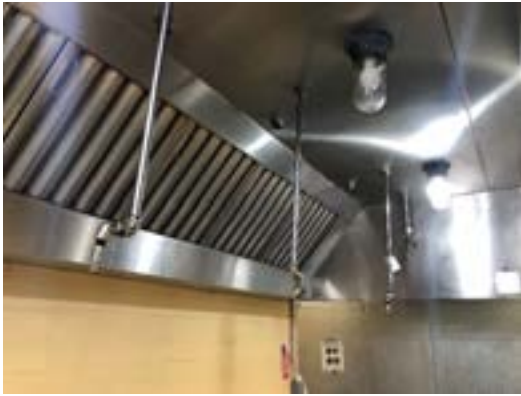
Kitchen Hood Suppression
