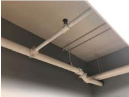
Upright Sprinkler & Piping
