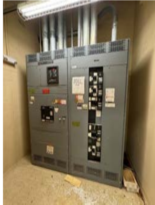
Switchboard #3 (480Y/277V, 2000A)
