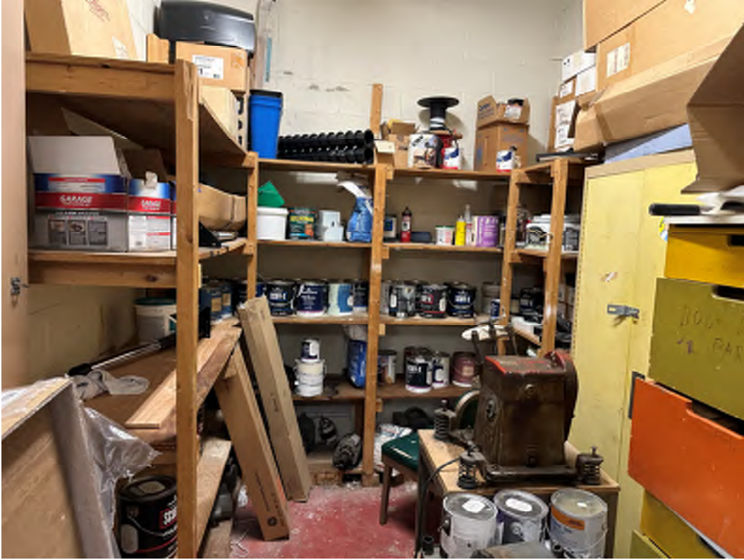
Photo 3: Paint storage in the boiler room.
