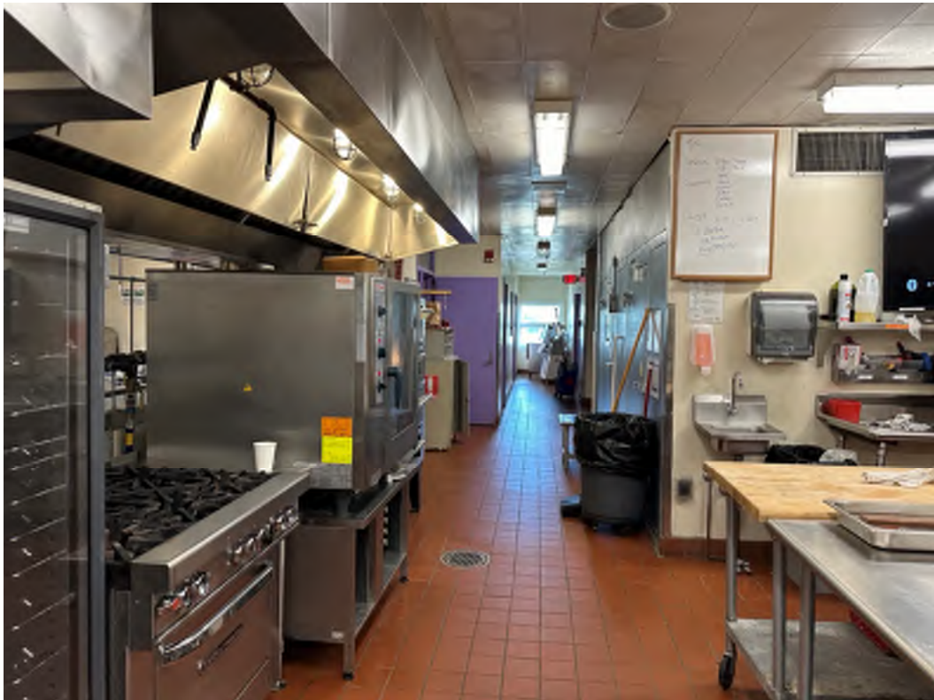
Photo 4: Floor drain observed in culinary arts kitchen.
