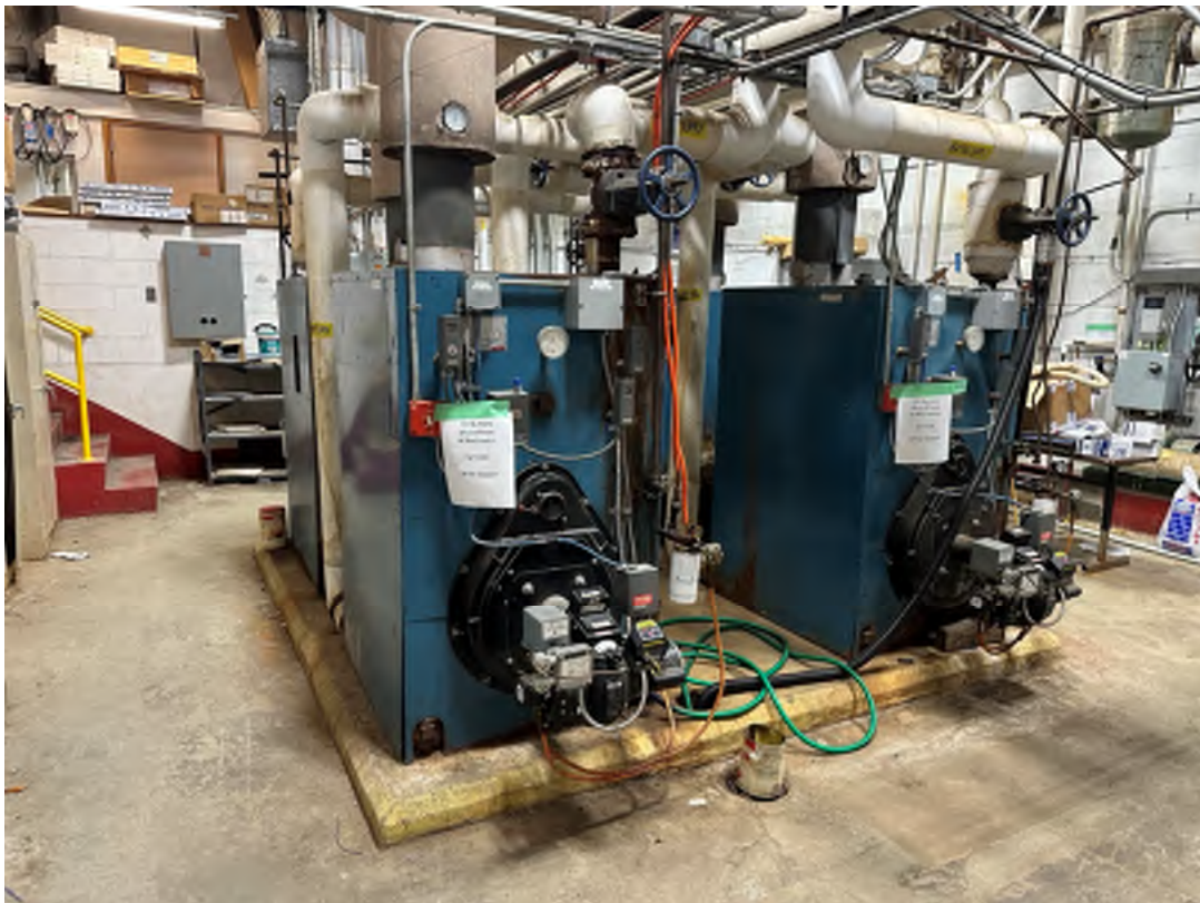
Photo 2: Boiler room with four oil burners.
