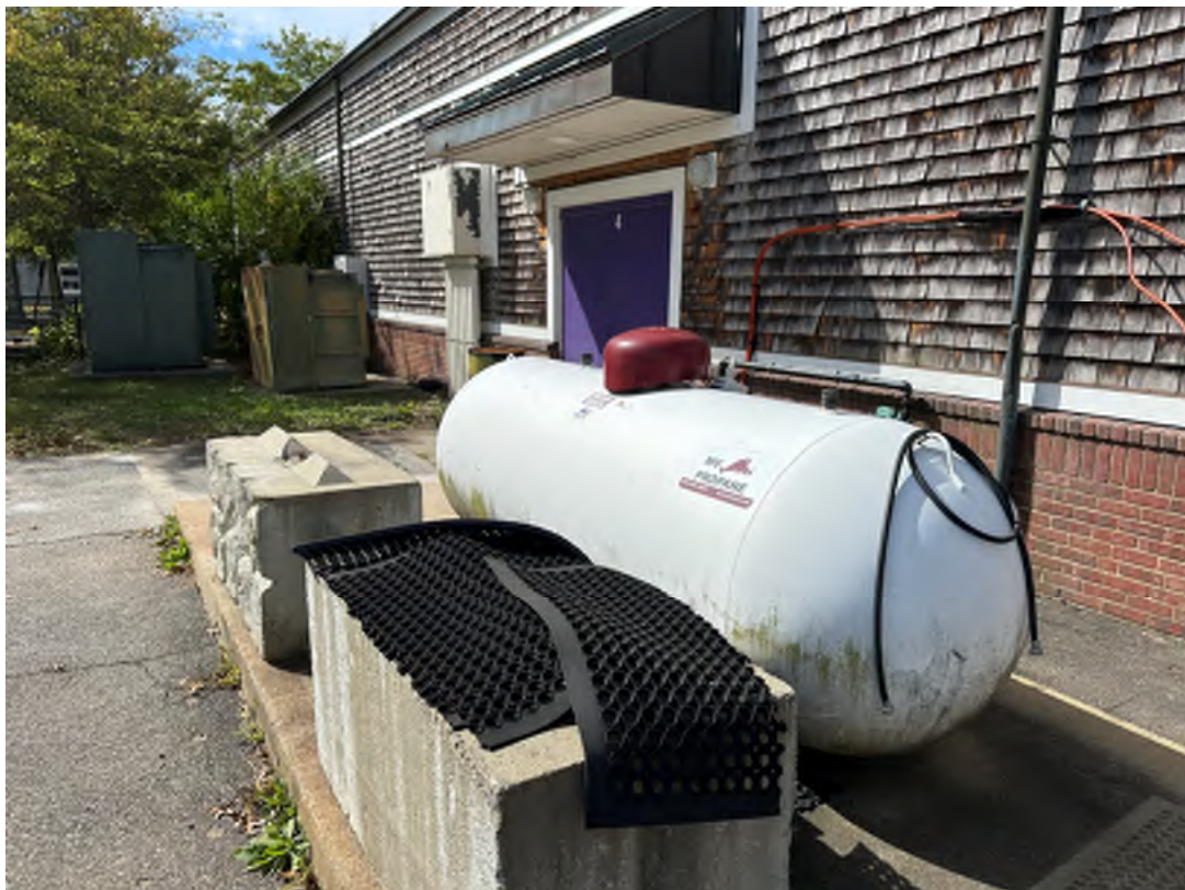
Photo 16: Large liquid propane tank located on eastern side of building.
