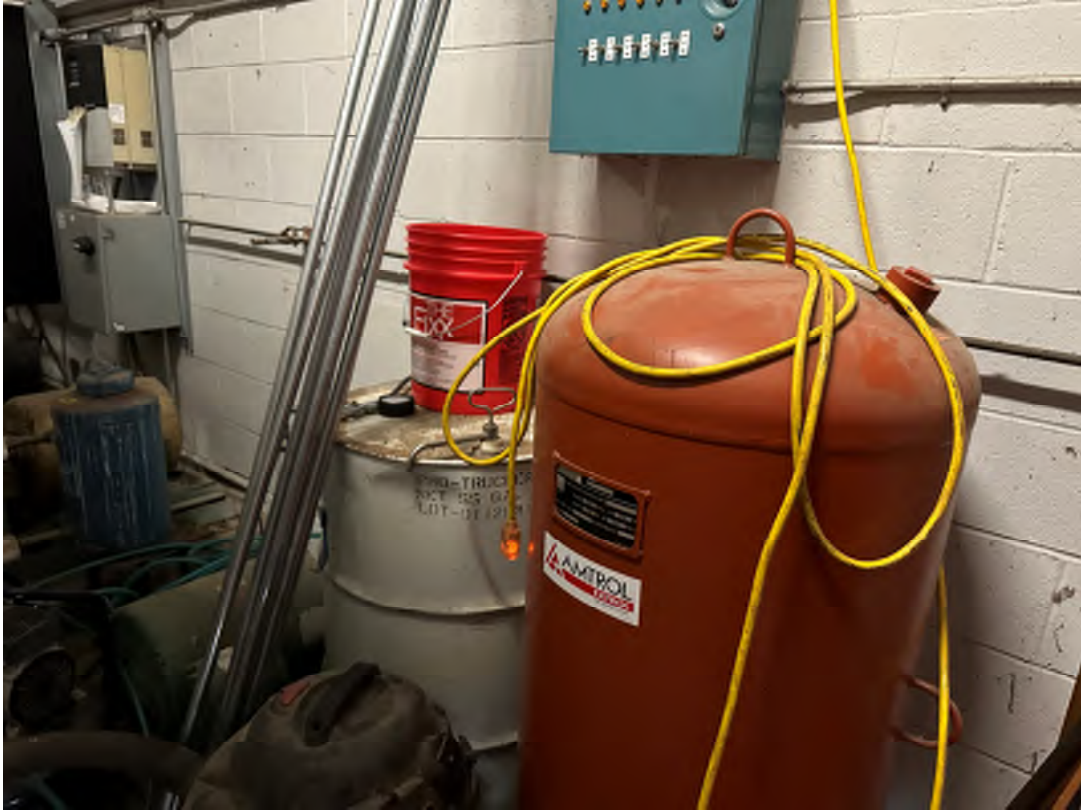
Photo 11: 55-gallon drum of unknown contents observed in boiler room.
