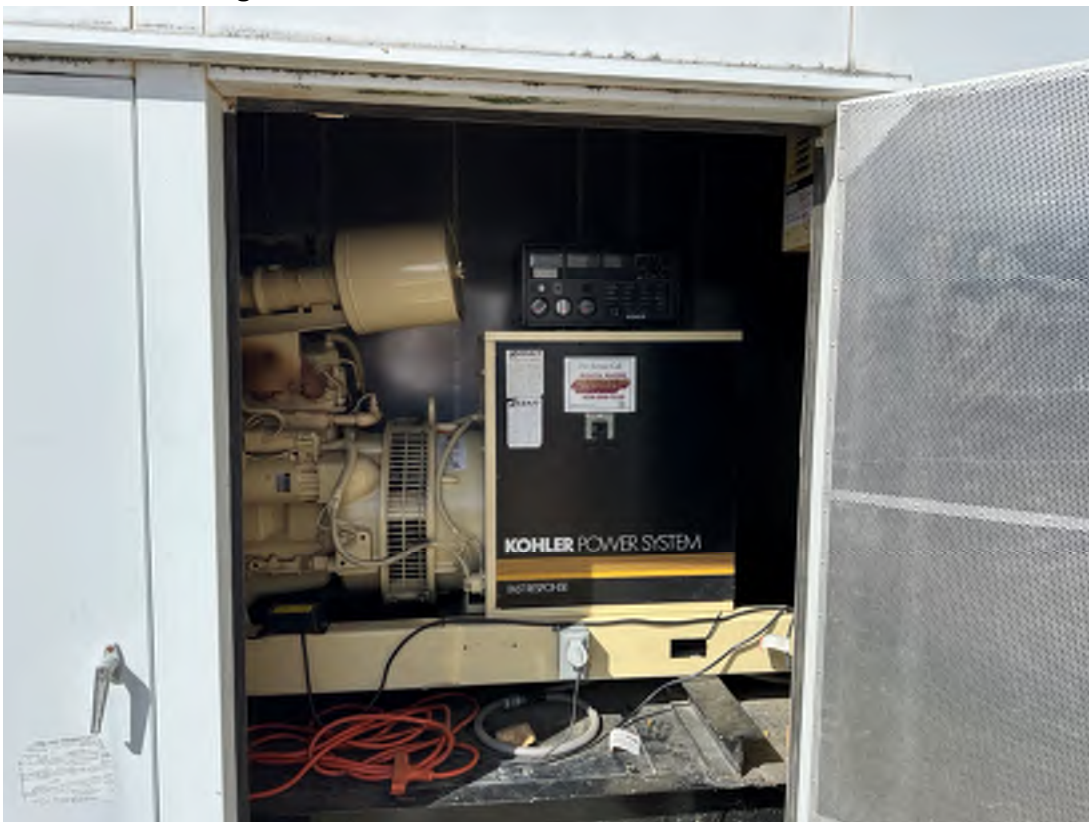
Photo 12: Backup power generator located outside boiler room.
