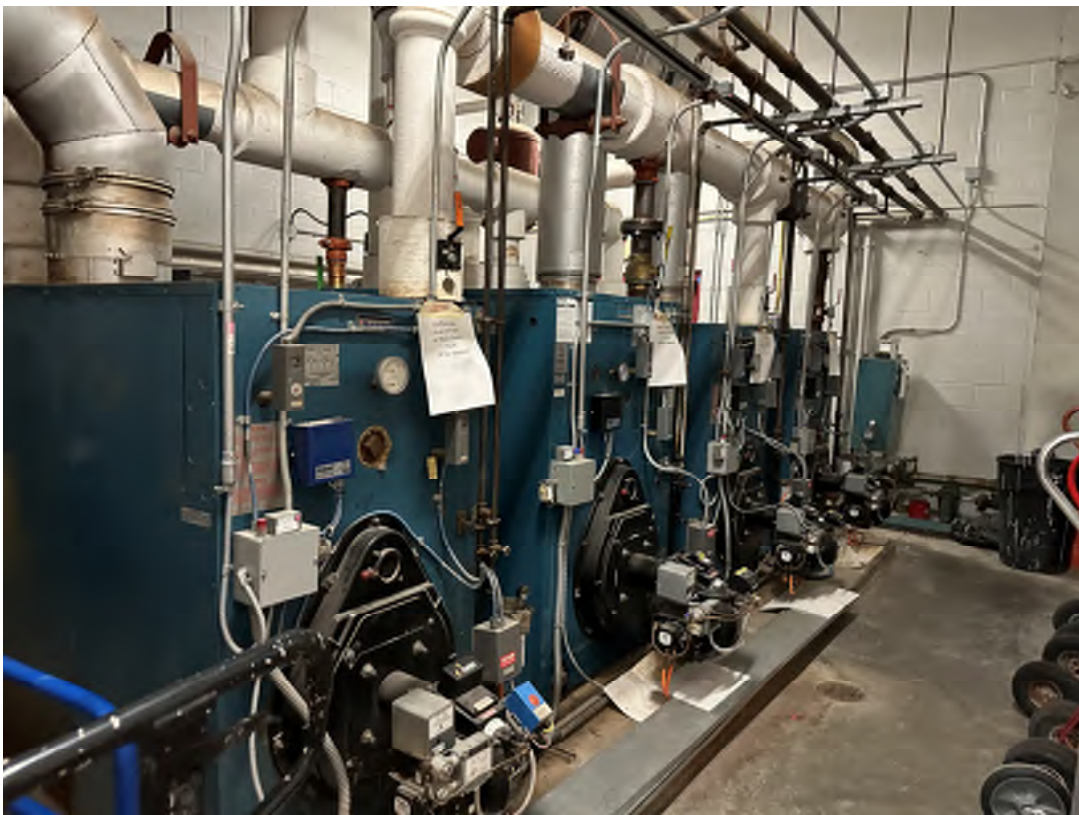
Photo 10: Second boiler room with four oil burners.
